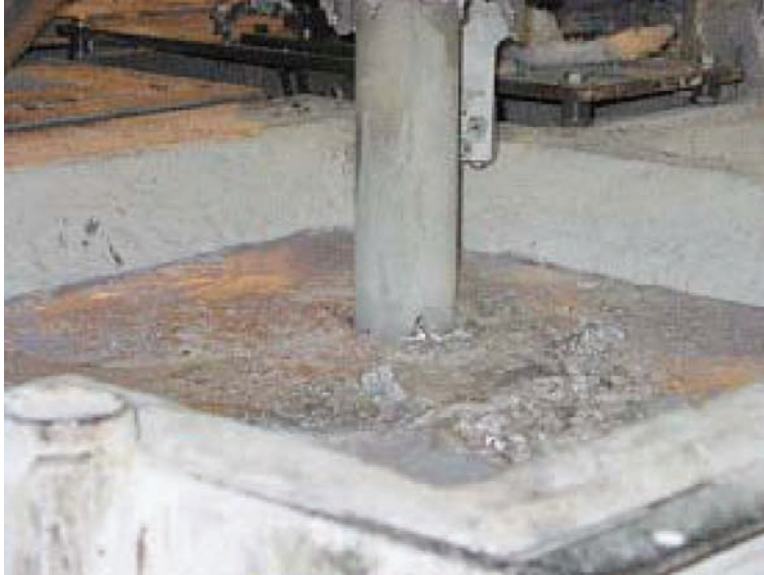
Figure 5: LIBS probe installed in Commonwealth's filter bowl [1].
