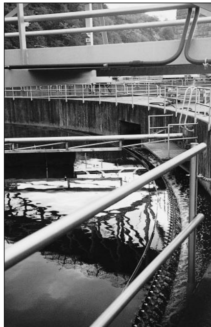
This is a close up of the weirs of the clarifier and shows the use of 316 stainless steel bolting.
