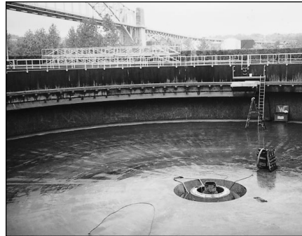
This photograph shows a secondary clarifier retrofit at a municipal wastewater treatment plant.
