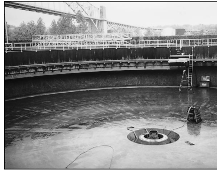
This photograph shows a secondary clarifier retrofit at a municipal wastewater treatment plant.
